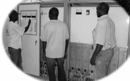
Nautel 100KW Transmitter
